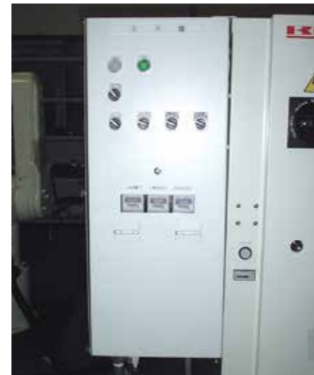
Painting unit control panel
